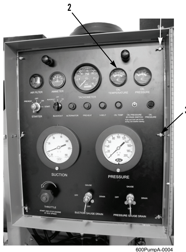
Figure 2. Oil Temperature Gauge at Control Panel.
