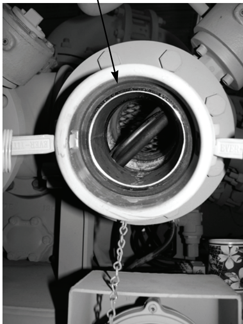
SUCTION INLET 600Pump-0121
