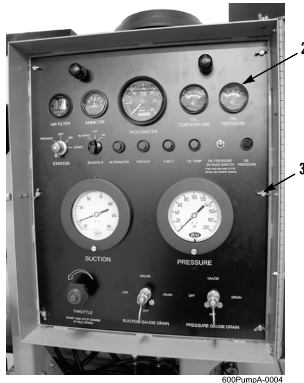
Figure 2. Oil Pressure Gauge at Control Panel.
