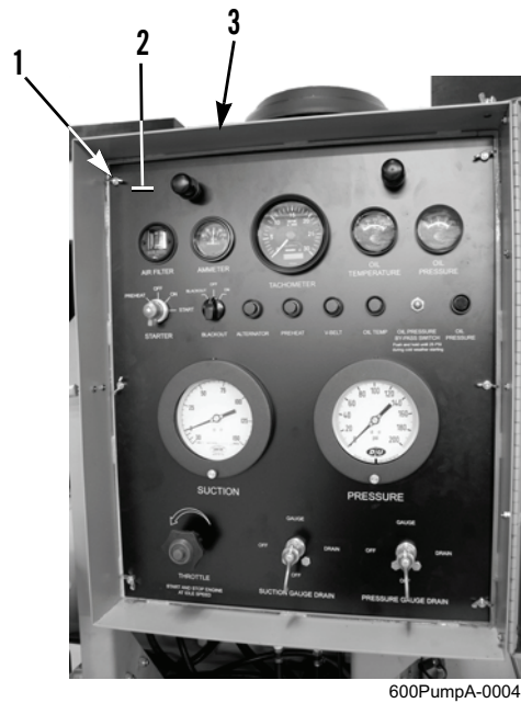
Figure 1. Control Panel Box.
